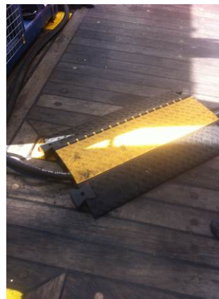
Fig.4.2.6.a - Cable protector (Photo UTM)
