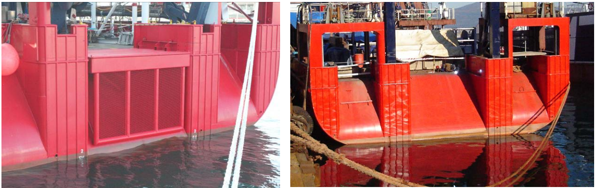
Fig. 4.2.6.1.d - Cover for stern ramp on R/V Sarmiento de Gamboa. (Photo CSIC) The vertical grating is to break waves.
